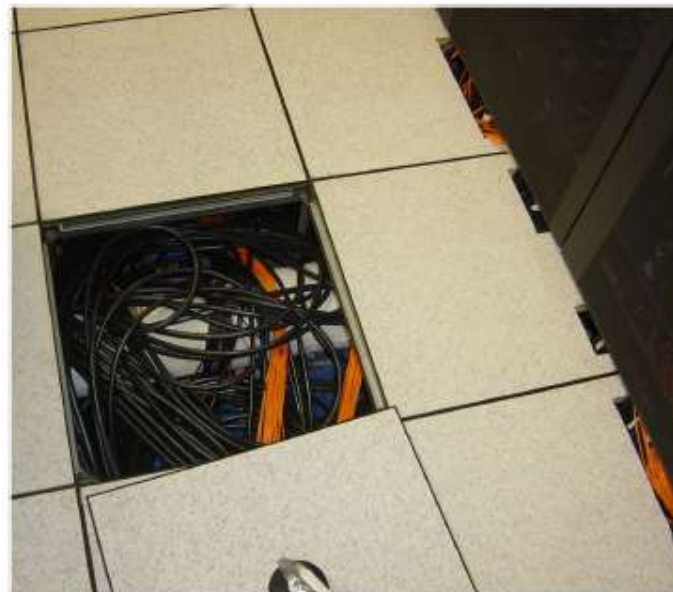
Figure 2.23 Under raised-access floor blockage.
