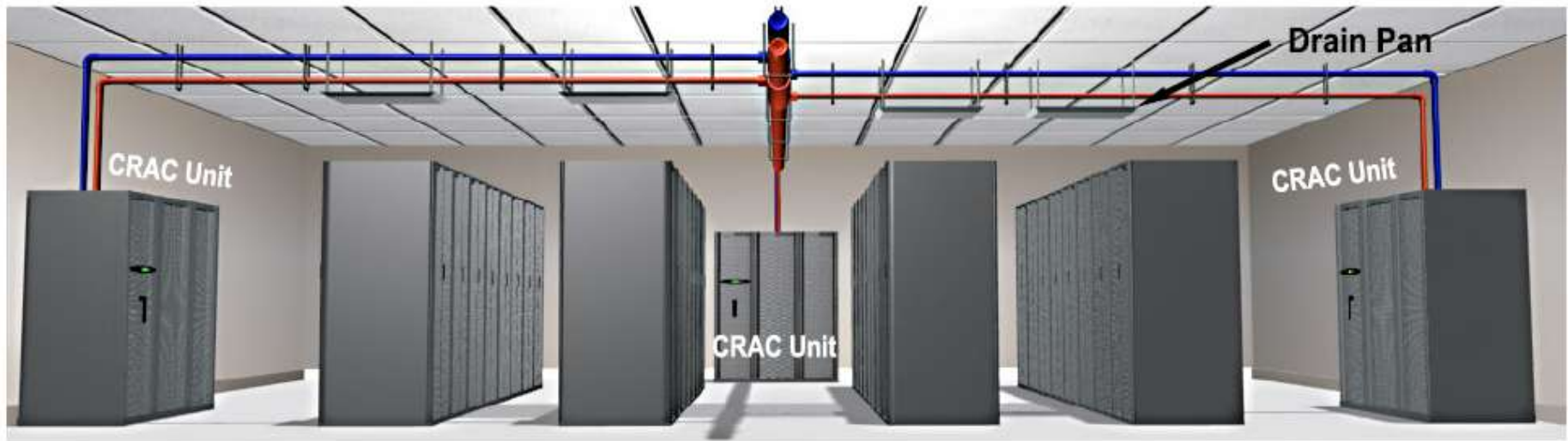
Figure 2 – Overhead piping with drain pan above racks.
