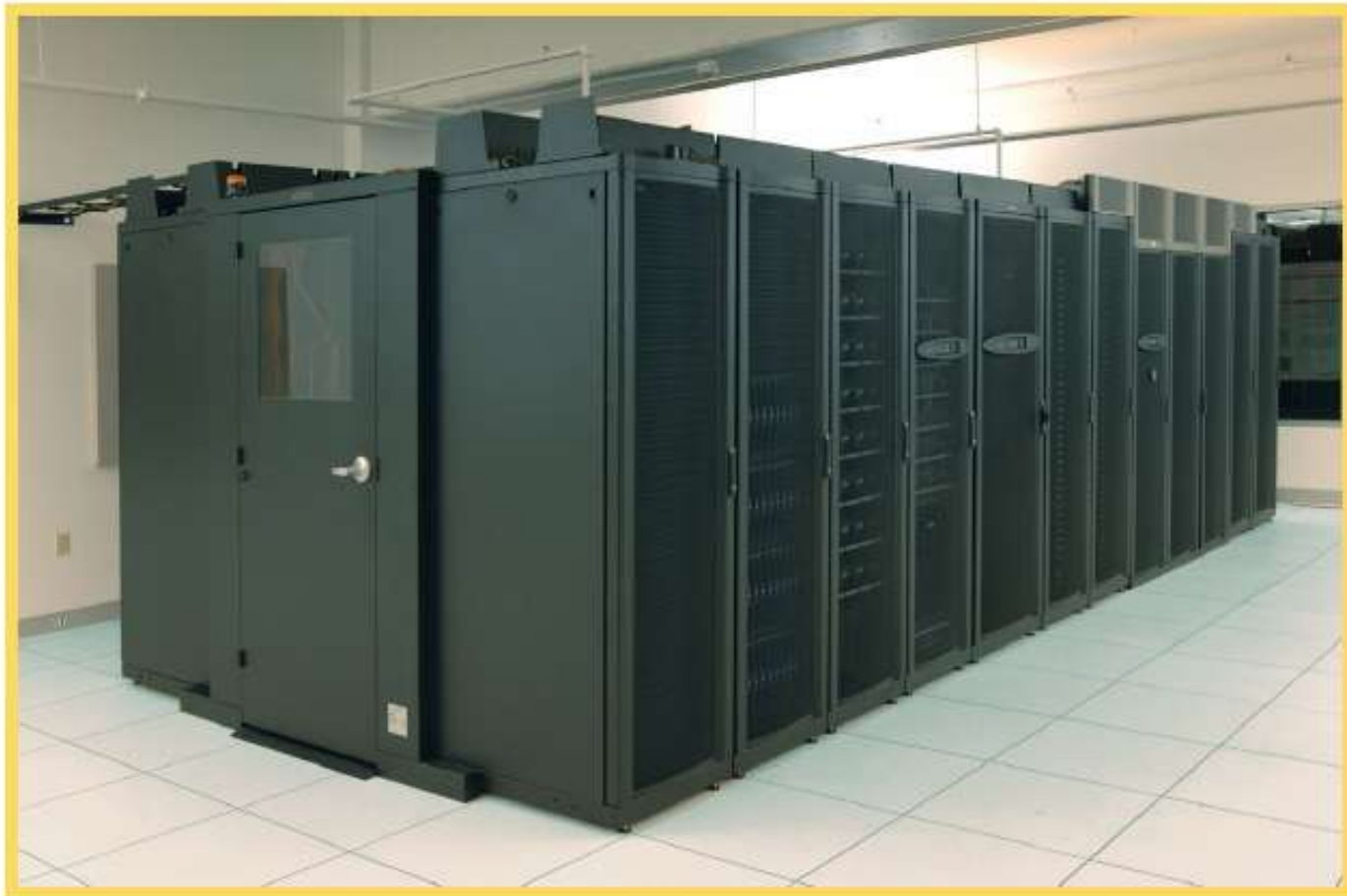
Figure 6 – Hot aisle containment system (HACS) operating as an independent zone
