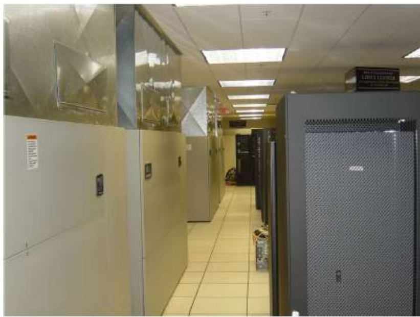
Figure 2.22 CRACs with return-air duct extensions.
